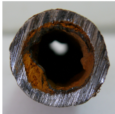
Fig. 1. Piping section with scale deposit
